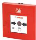
Manual Pull Station
