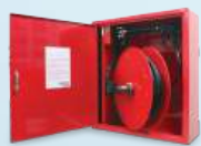
Fire Hose Cabinet
